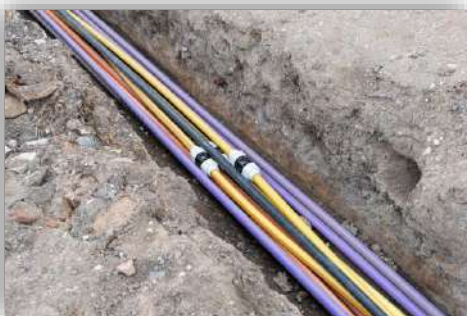
Underground Electric Transmission Lines
