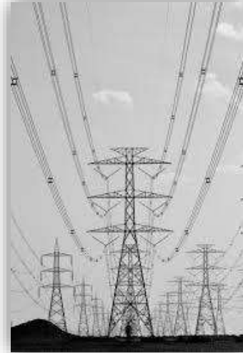
Overhead transmission lines
