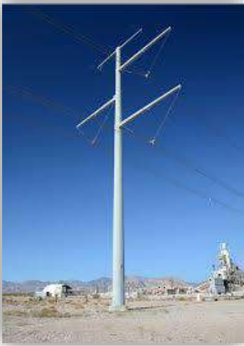
Transmission Line using Monopoles
