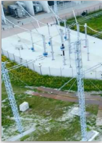
Emergency Restoration System
